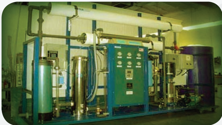
Industrial R/O Systems
